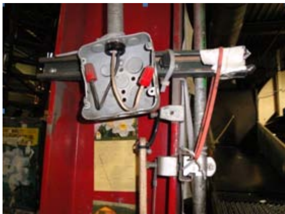
Exposed Electrical Wires, [REDACTED]
