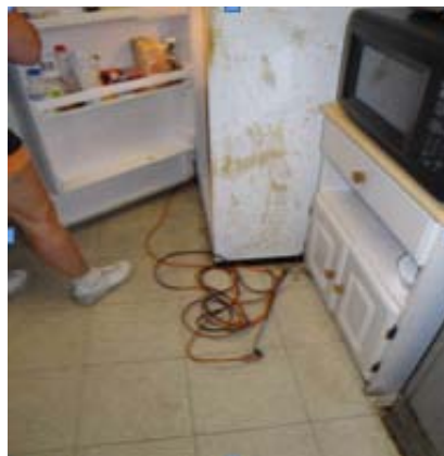
Extension Cord Used in Lieu of Permanent Wiring, [REDACTED]
